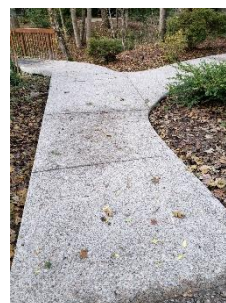
New sidewalk at the East Bridge next to 40 Brae Burn Drive – the Big Bridge.
