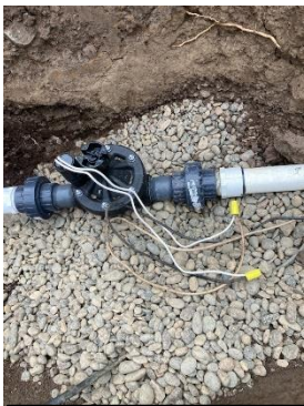
Irrigation valve in front of 8 Westbrook Way
