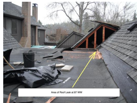
87 WW Roof Leak
