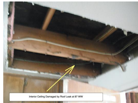
87 WW Ceiling Damage
