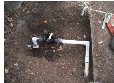
New Irrigation Valve at 198 BB
